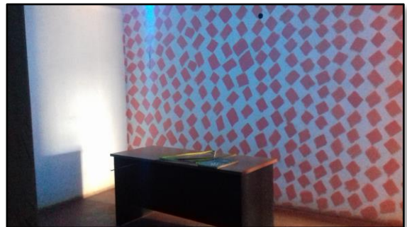
FUTURE: Classroom #1 (Needs some wall repair...and repainting!)
